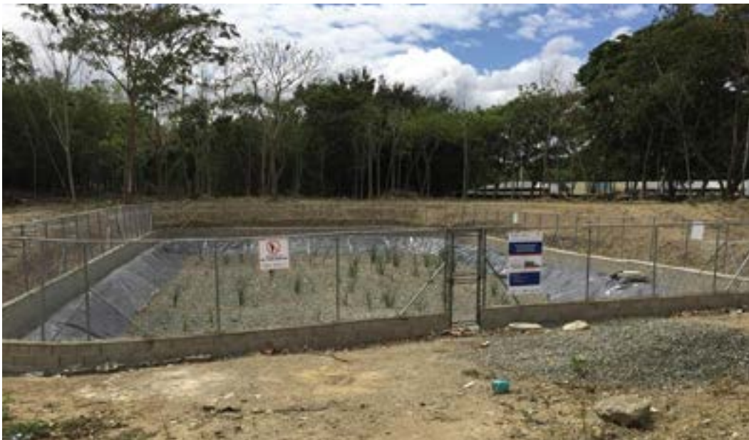
Figure 2: To reduce vulnerability of communities during tropical storms and hurricanes, USAID improved the collection and treatment of wastewater using techniques such as this constructed wetland in Santiago.
