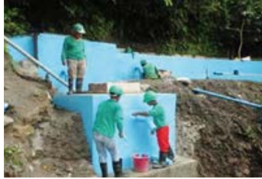
Photo credit: Kananga Waterworks.
